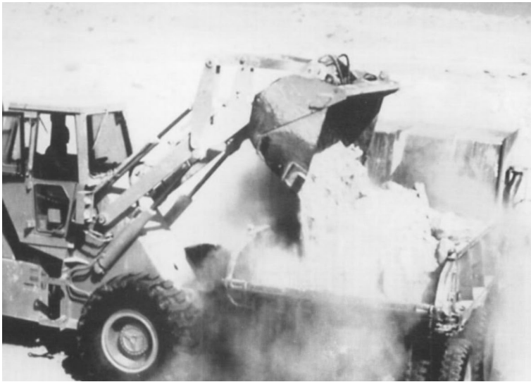
GSG-2 engineers dig and transport marl to stabilize the soil at Jubayl Naval Air Facility. (Photo by LtGen James A. Brabham, Jr.)
